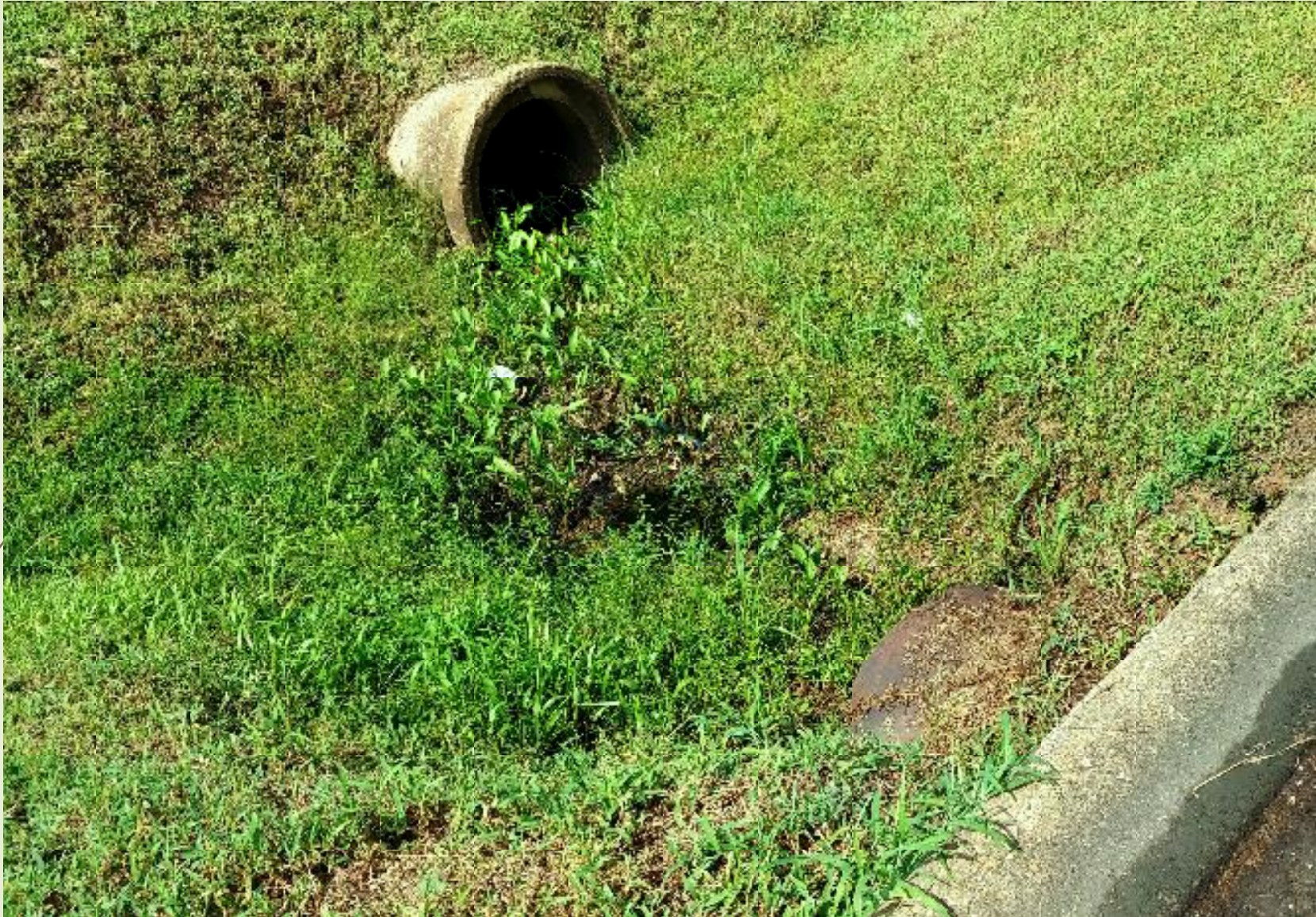
Culverts under Mission Dr. and Ehrhardt Park sidewalk
